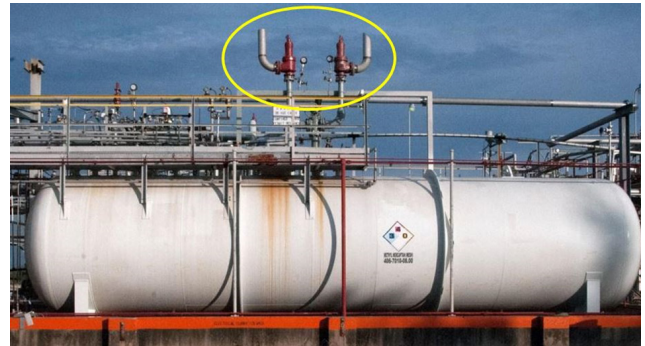
Figure 3. DuPont’s uninsulated methyl mercaptan storage tank. Pressure-relief valves relieving to the atmosphere are circled in yellow.
