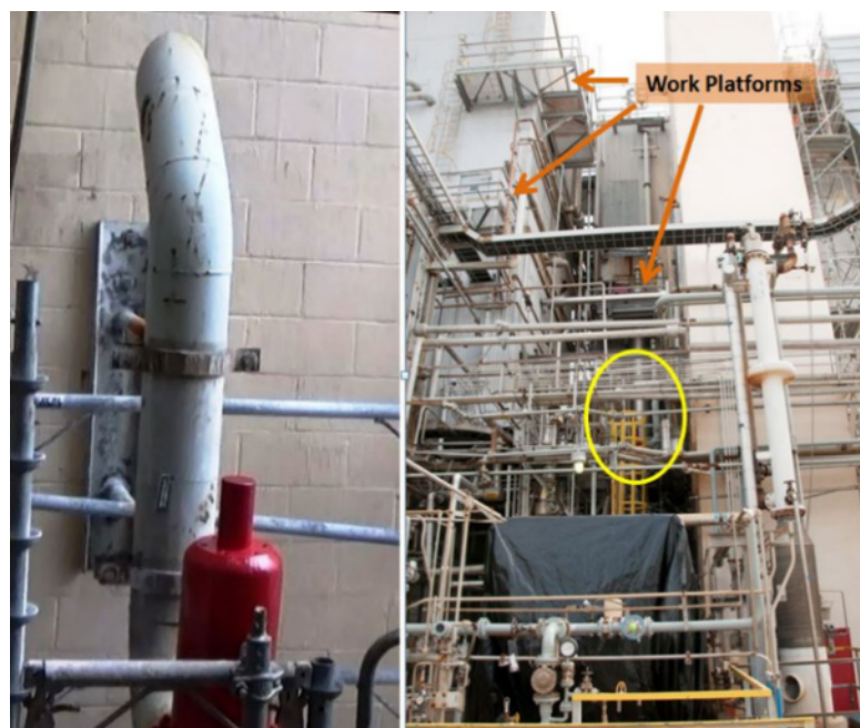
Figure 6. Chlorine gas discharged from this pressure-relief system below work platforms and in a congested area at DuPont. The relief valve location is circled in yellow.
