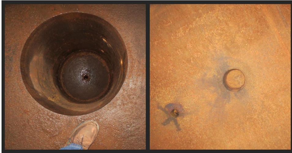
Figure 26. Photos of the Final Fractionator Overhead Accumulator taken during TPC PNO's 2017 turnaround. (Credit: TPC)
