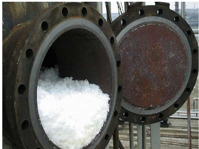
Figure 4. Popcorn polymer in a manway from an undisclosed facility (Credit: International Institute of Synthetic Rubber Producers Inc. [8, p. 261])
