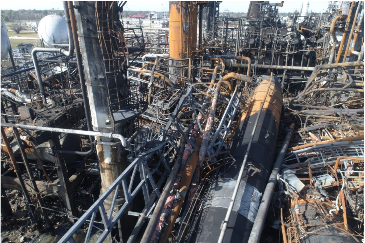
Figure 15. Damaged piping and equipment in the South Unit. (Credit: TPC)
