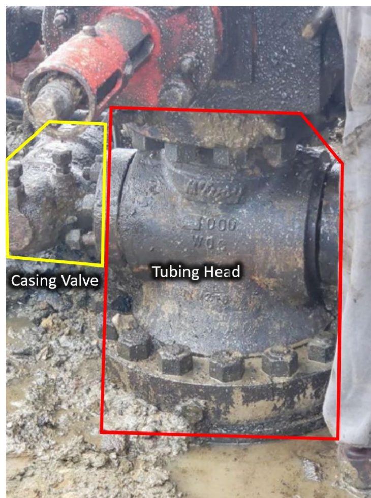
Figure 13. Existing tubing head with one of the casing valves attached. (Credit: Chesapeake, annotation by CSB)
