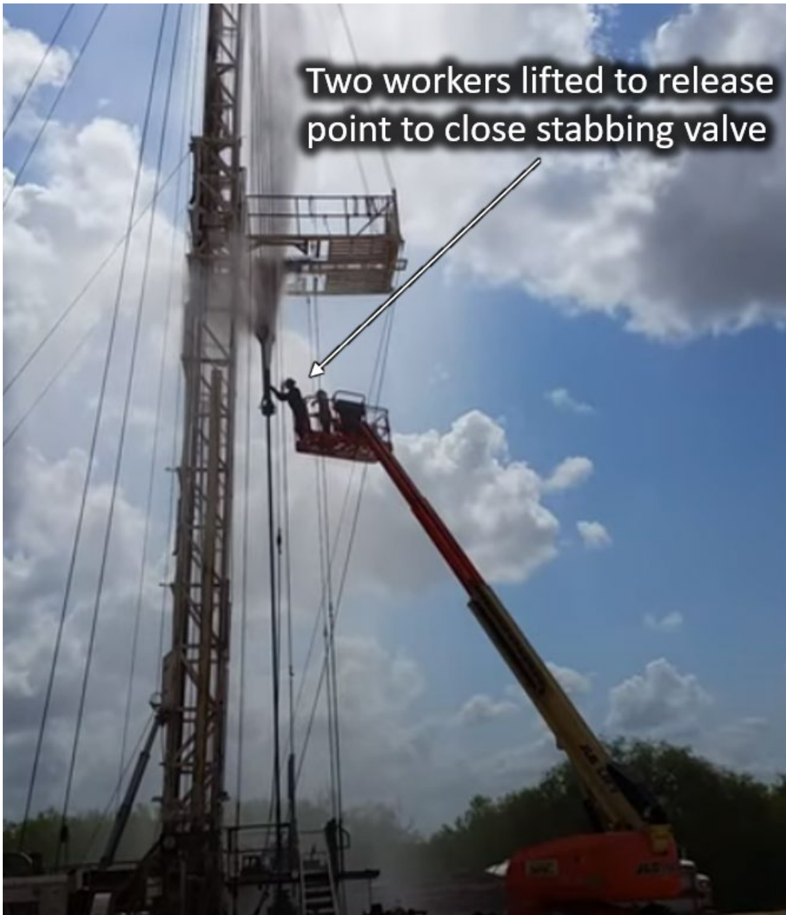
Figure 27. Two workers closing a stabbing valve following a blowout. (Credit: YouTube [27], annotation by CSB)
