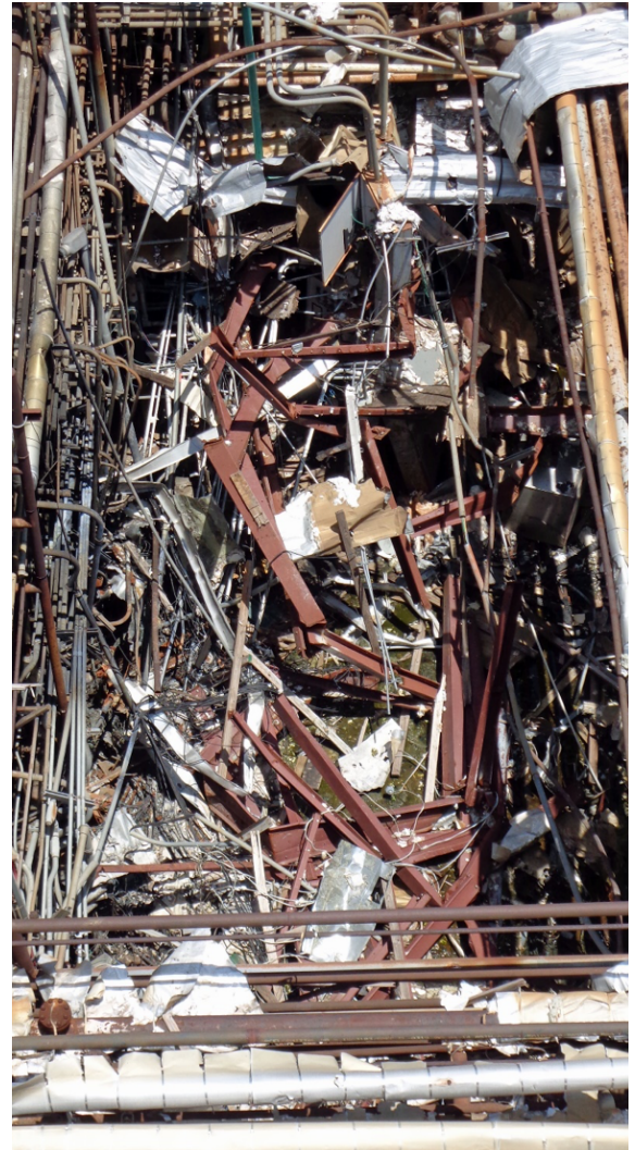
Figure 8. Plant Building (Top View). This photo, taken from the top of adjacent equipment, shows the post-incident condition of the plant building. (Credit: CSB).
