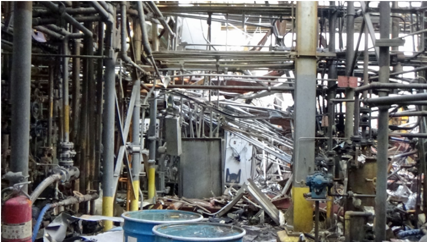
Figure 6. Plant Building (North Side). This post-incident photo shows the path KMCO workers commonly took to enter the plant building. With process units on the left and right, this walkway led to the entrance on the north side of the plant building, where emergency responders recovered the operator. (Credit: CSB).
