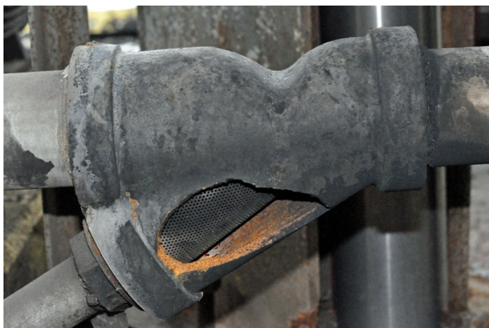
Figure 11. Y-Strainer. This photo shows west side of the failed y-strainer involved with the April 2, 2019 incident. (Credit: CSB).
