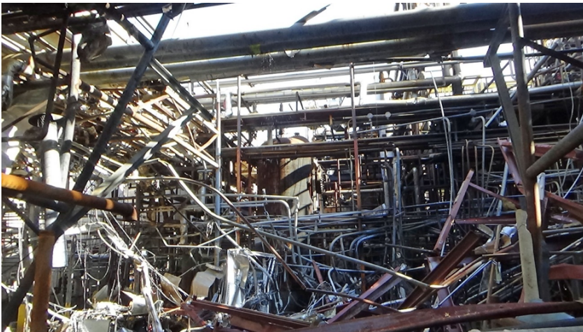
Figure 7. Plant Building (South Side). This post-incident photo shows the south side of the plant building. (Credit: CSB).
