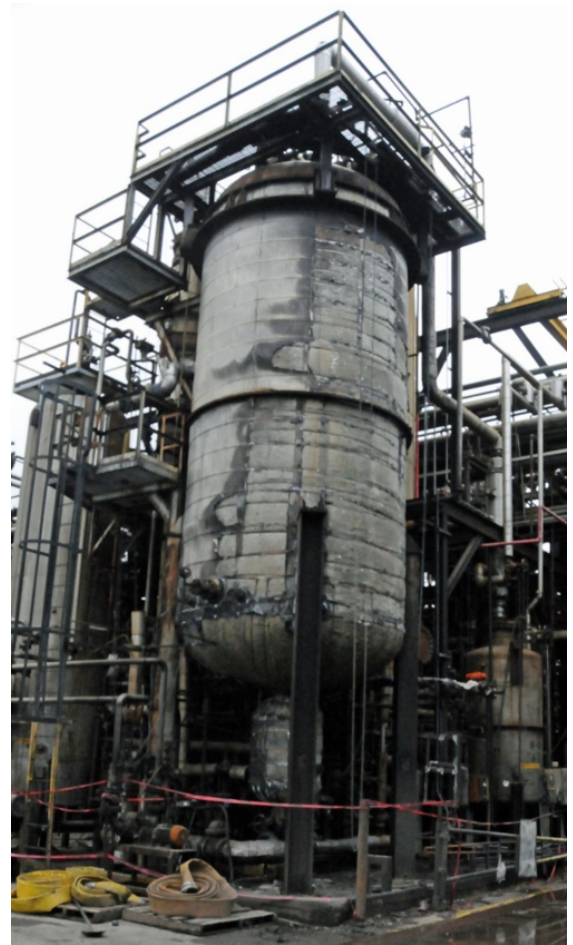
Figure 3. Batch Reactor. This photo shows the post-incident condition of the batch reactor KMCO used to manufacture sulfurized isobutylene products. (Credit: CSB).
