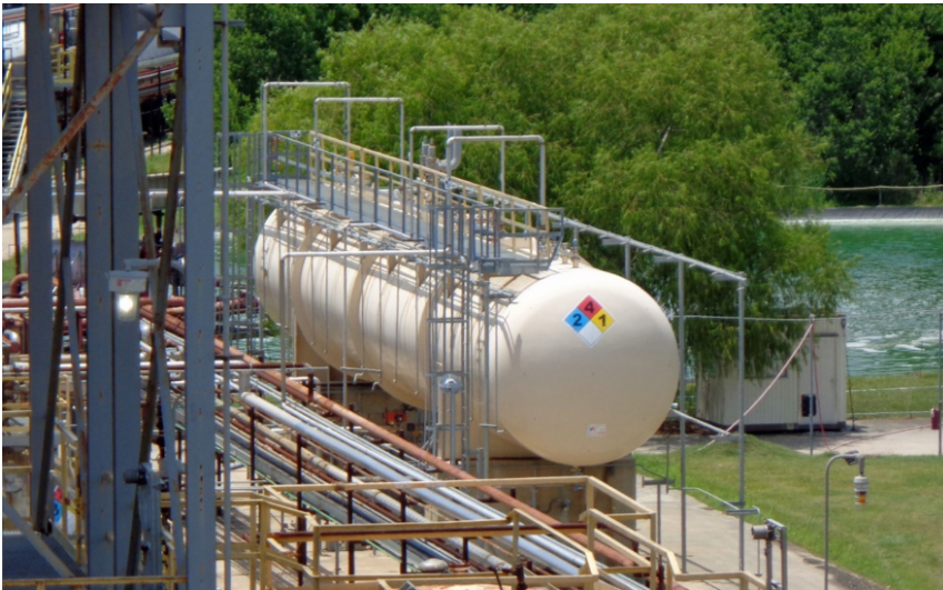
Figure 2. Isobutylene Storage Tank. KMCO's 70,000-gallon isobutylene storage tank was built in 2014 and the tank was commissioned and began operating in 2015. The tank is made from SA-516-70 carbon steel, has an inner diameter of 12 feet, and is 80 feet long (seam-to-seam). The tank's 2:1 elliptical heads add to the overall length. The maximum allowable working pressure is 200 pounds per square inch at 150 degrees Fahrenheit. The isobutylene storage tank was designed to meet the 2013 edition of the American Society of Mechanical Engineers (ASME) code, Section VIII, Division 1. (Credit: CSB).
