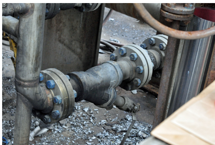
Figure 10. Y-Strainer (East Side). This post-incident photo shows the top and east side of the three-inch y-strainer on the inlet piping to the isobutylene charge pump. The orientation of the y-strainer was such that the straight through flow was headed north. (Credit: CSB).
