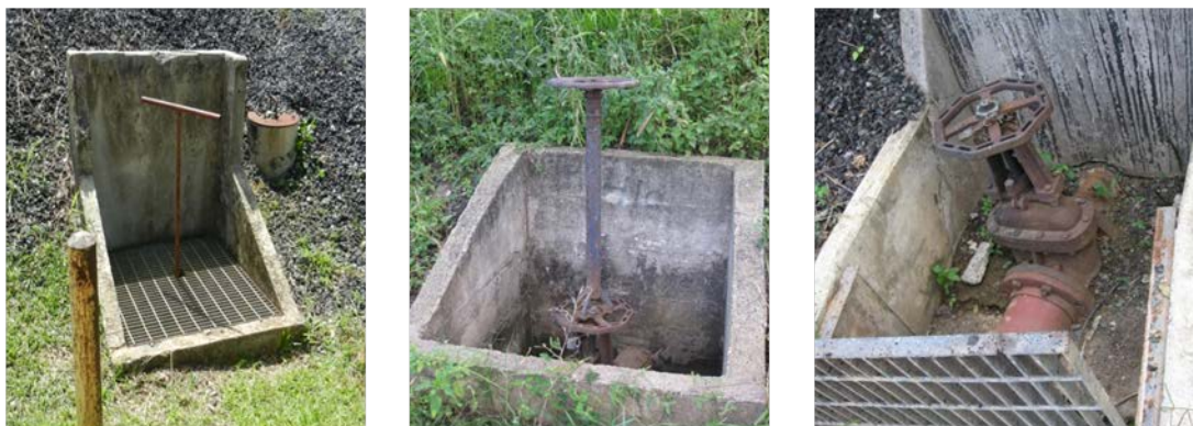
Figure 15: Various dike drain valves at CAPECO. Tank 409 dike drain valve (left): position of the valve is undeterminable without physically turning the valve. Rising stem valves (center, right). In some cases, the valve position is hidden in the sump (center).
