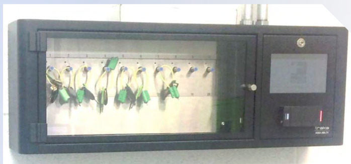
New key fob lockout system (photo courtesy of MGPI)
