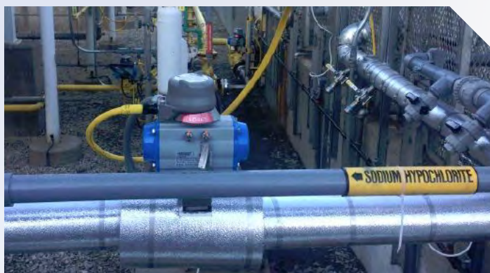
New shutoff valve (photo courtesy of MGPI)
