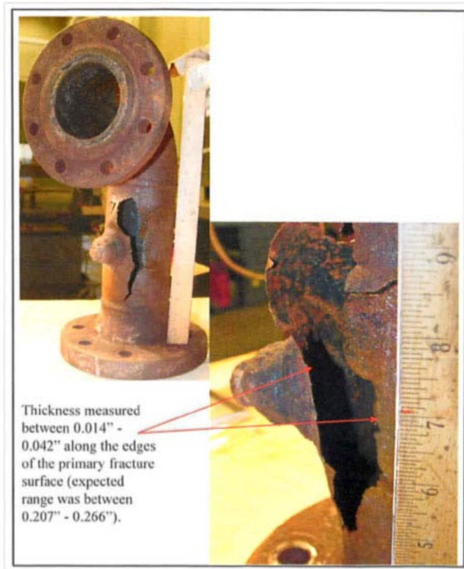
Figure 13. Failed piping component that resulted in the 2007 Richmond crude unit fire. This carbon steel piping was found to contain less than 0.005 percent silicon.
