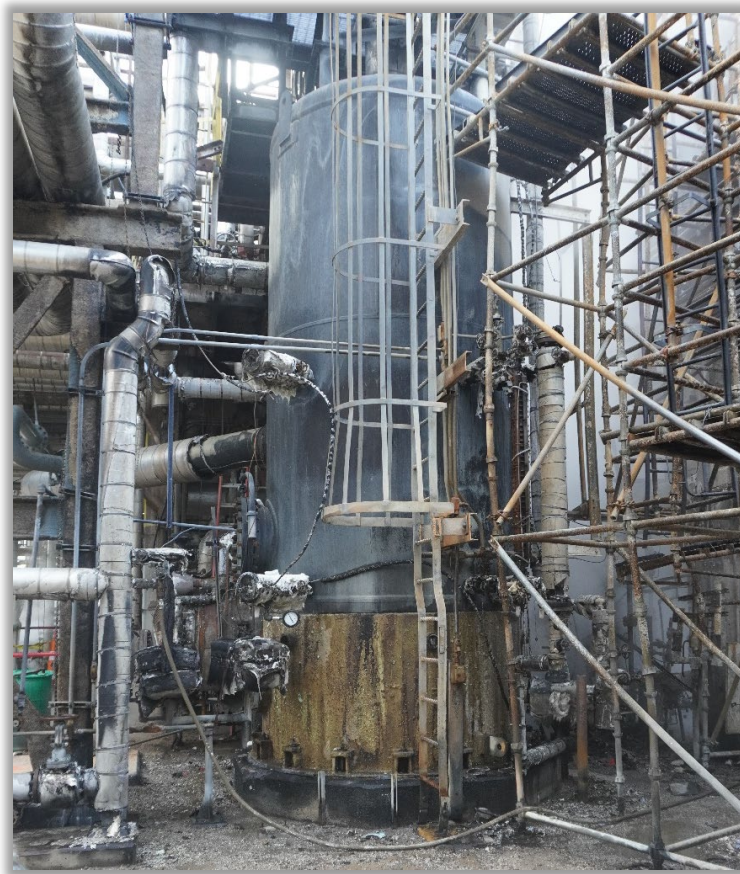
Figure 1. Fuel Gas Mix Drum at the BP-Husky refinery. (Credit: CSB)
