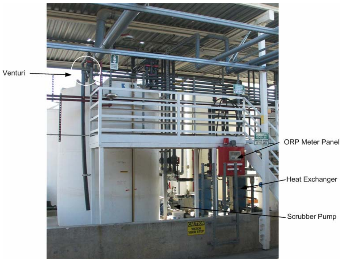
Figure 5. Caustic scrubber (typical)
