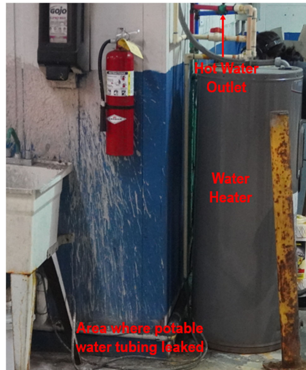
Figure 24. Location of polyethylene line that leaked, causing an area in the Bio-Lab Conyers Plant 6 to flood. (Credit: CSB)
