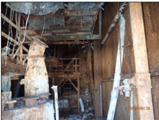
3 rd floor level from north stair, showing heat-deformed columns & bracing (Atlas, 9/29/2020)
