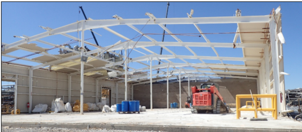
Eastern bay of south FGW, looking SW. Wrecked framing has been removed (Atlas, 9/29/2020)
