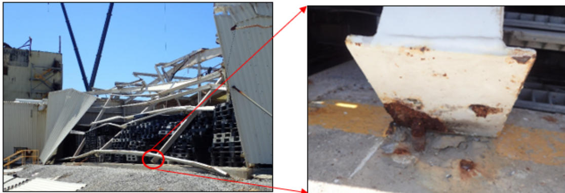
Eastern bay of north FGW, looking SW, & close-up of column base and anchor bolts (Atlas 9/29/2020)
