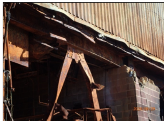
Ground floor level looking east, showing heat-deformed brace & spandrel (Atlas, 9/29/2020)
