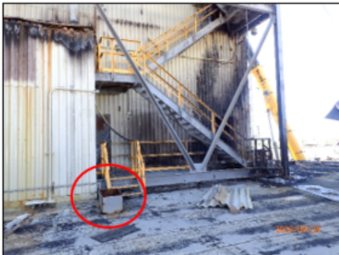
Roof opening at broken duct, Low Bay roof north of High Bay tower (Atlas 9/29/2020)
