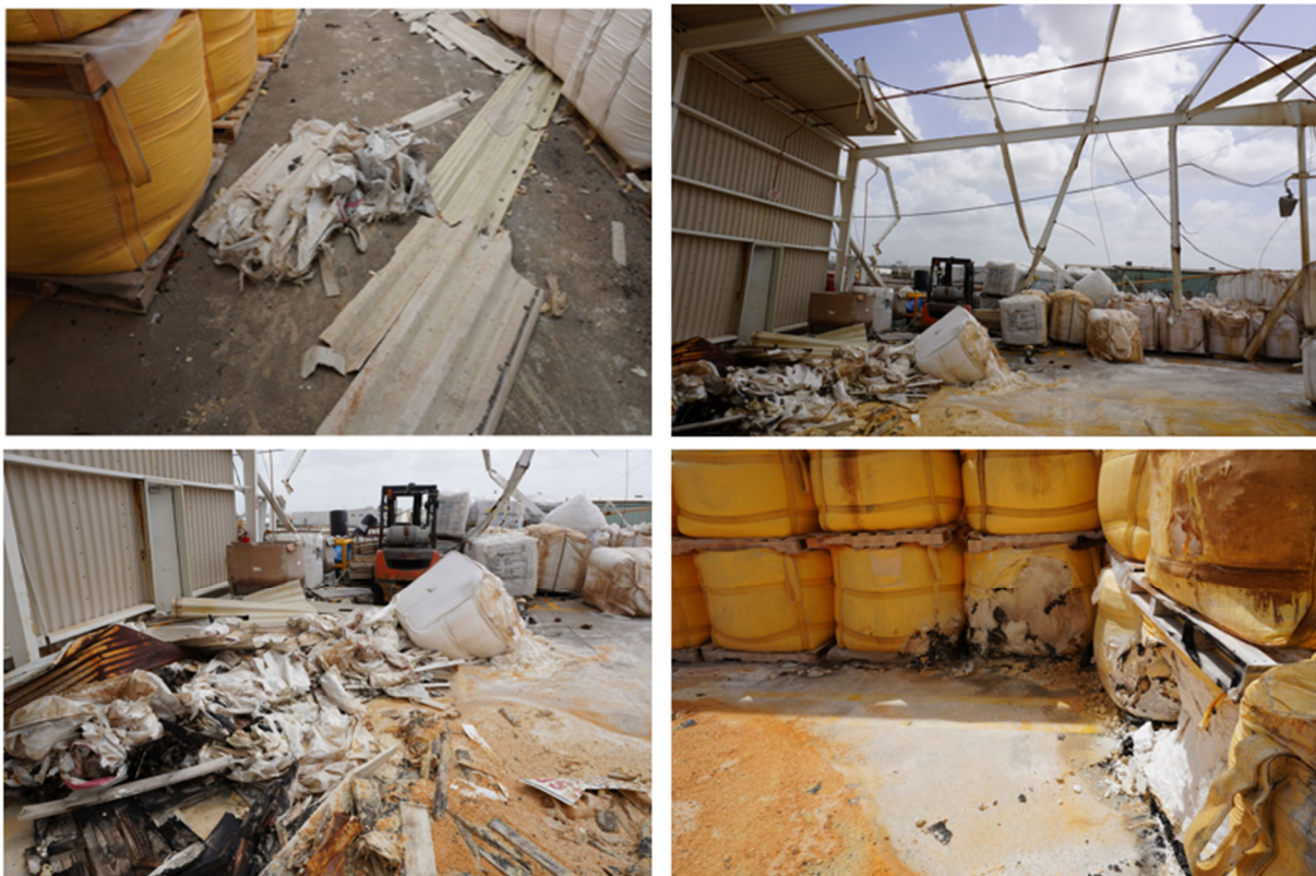
Figure 14. Inventory and storage areas inside the Finished Goods Warehouse following the second event. (Credit: CSB)
