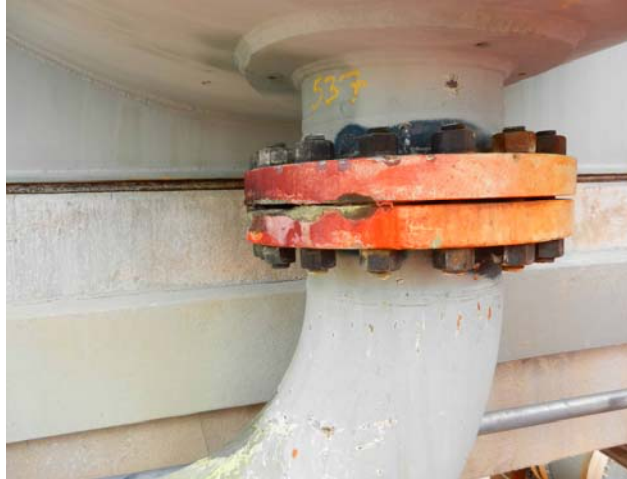
View of the flange involved in the HF release at the CITG Corpus Christi Refinery
