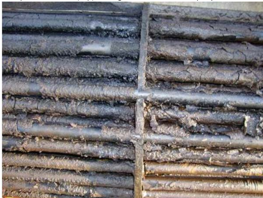
Example of hot shell (top) fouling in API member company NHT Unit
