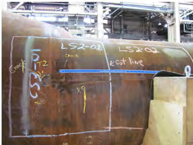
Marking on shell- note tee at T2 location
