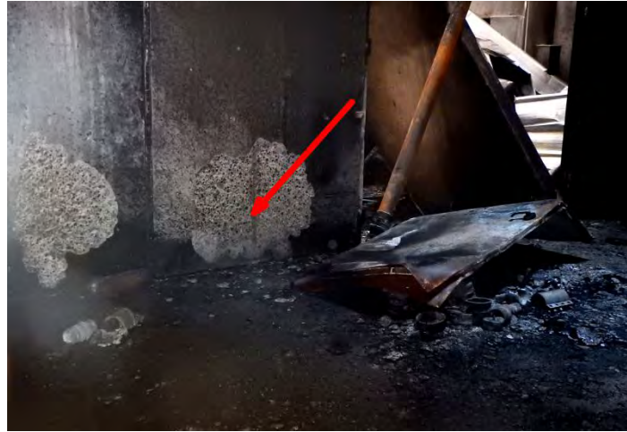
Figure 3-37. Example of High Fire Damage Indicator (Spalled Concrete)
