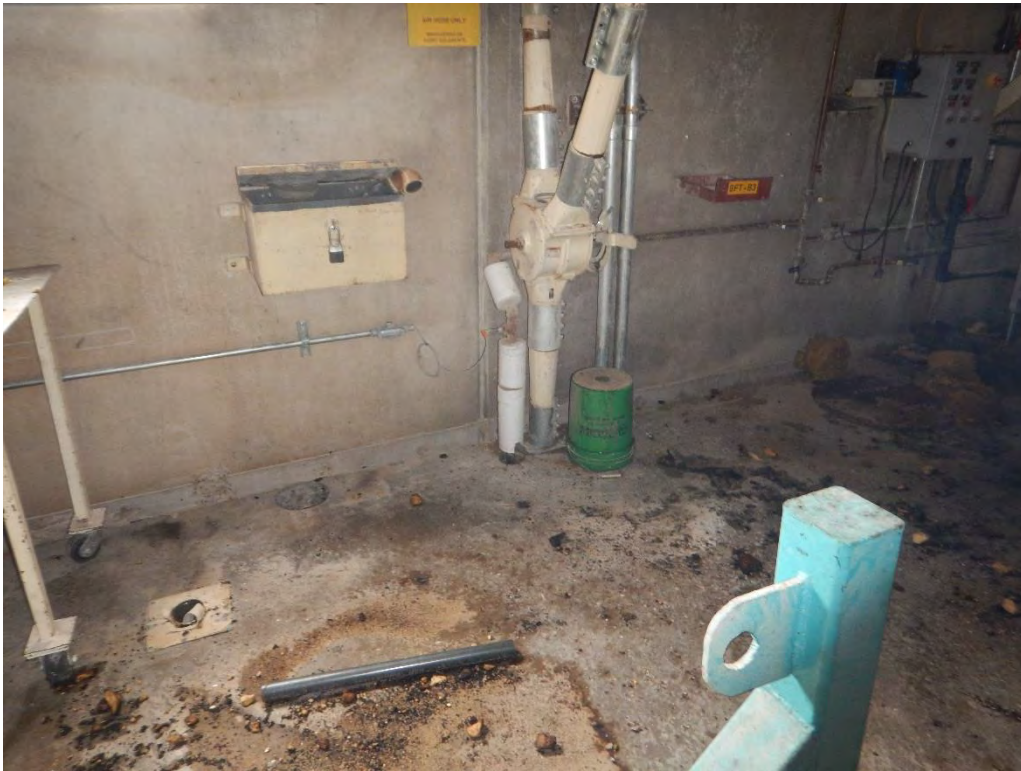
Figure 2-3. Mill B Wall Panel to Level 2 Slab Connection Failure Perspective
