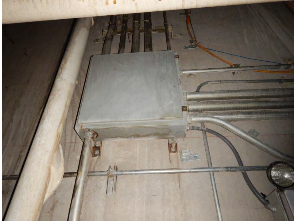
Figure 4-5. Mill B Undamaged Electrical Junction Box
