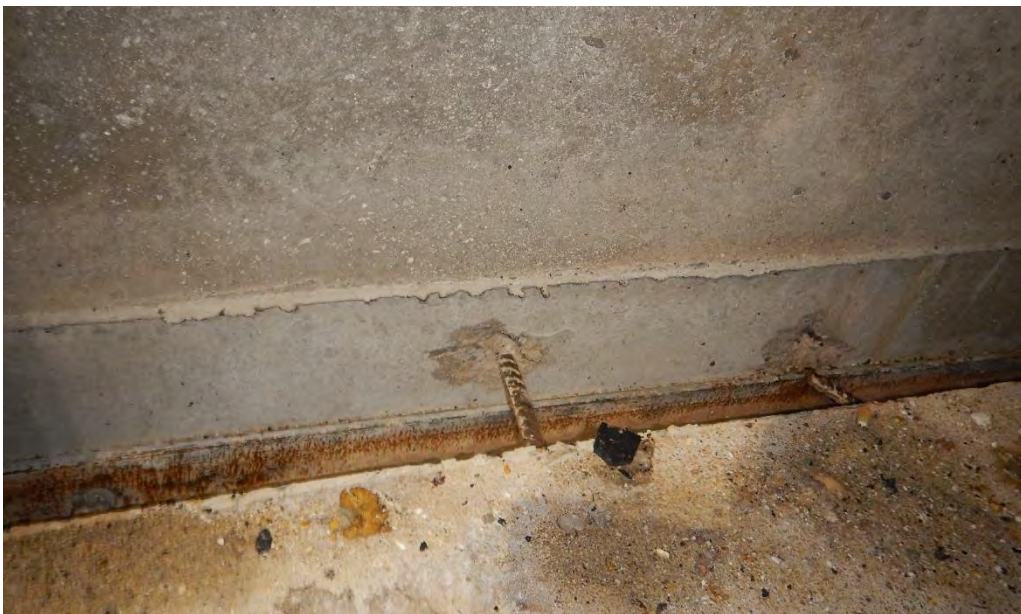
Figure 2-4. Mill B Wall Panel to Level 2 Slab Connection Failure Detail
