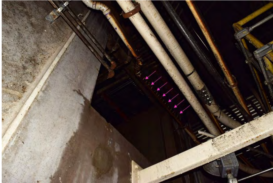
Figure 3-7. Mill B Level 1 Air Shaft Opening Fire Directional Indicator
