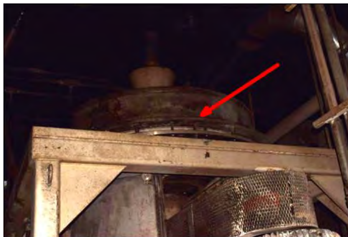
Figure 3-36. Example of Medium and High Fire Damage Indicator (Bubbled and Lost Coating)
