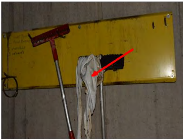
Figure 3-35. Example of Low Fire Damage Indicator (Melted Plastic)
