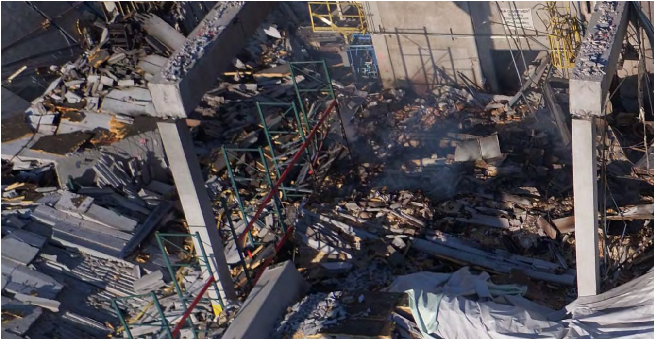
Figure 2-14. Failed Multipurpose Building Beam to Column Joint
