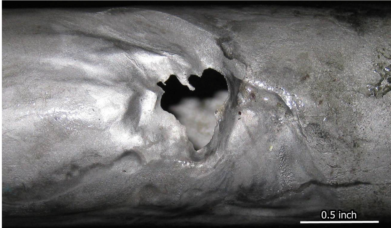
Figure 10. The larger hole eroded from the outside-in on the oleum sample line 26
