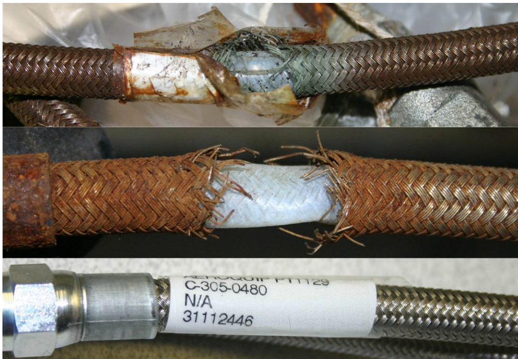
Figure 16. Flex hose comparison photographs: (top to bottom) ruptured riverside hose, flow restricted hillside hose, a new hose with attached ID tag
