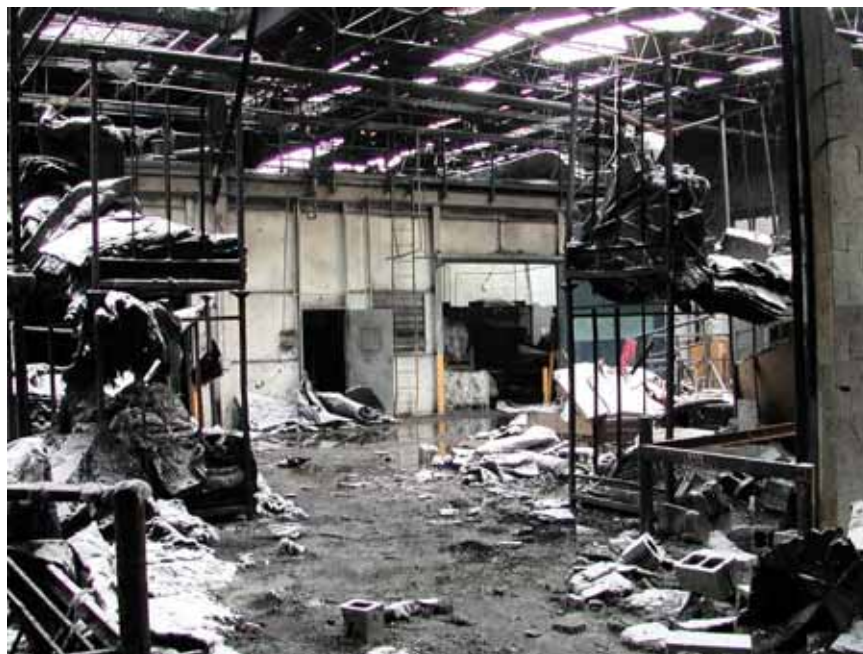
Figure 5. CTA Acoustics' production area after resin dust explosions 15
