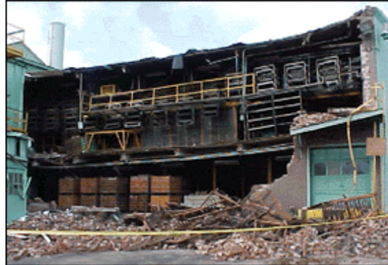
Figure 9. Shell mold building after Jahn Foundry Explosion (Springfield, Massachusetts, February 25, 1999). 21
