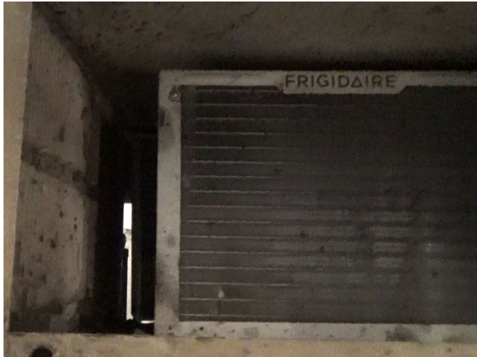
Figure 21. Wall-Mounted Air Conditioner. This photo, taken from outside of the PPE Room, shows an opening to the inside of the PPE Room. (Credit: CSB)
