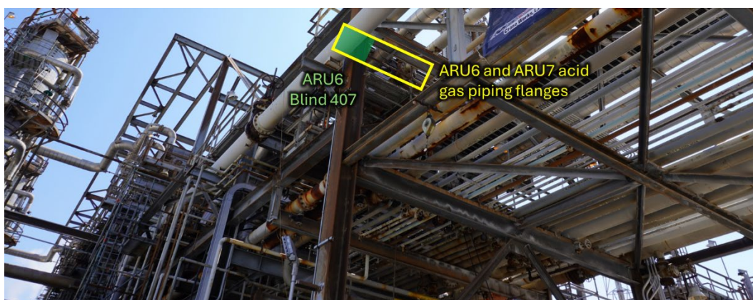
Figure 4. View of Blind 407 from the ground. (Credit: CSB)
