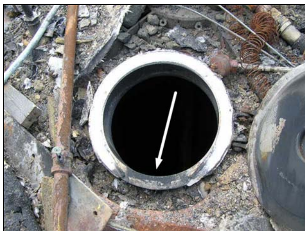
Figure 6. Damaged manway gasket, showing vapor release path
