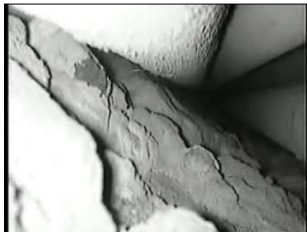
Figure 7. Deposits fouling the water side of the M1 reactor's condenser.
