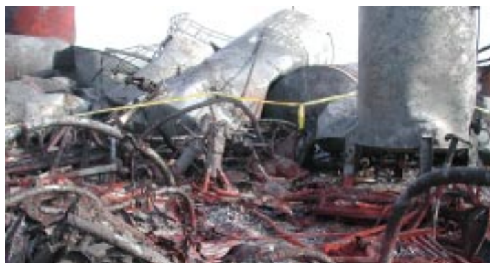
Figure 7. Collapsed blend tanks located near warehouse 1.
