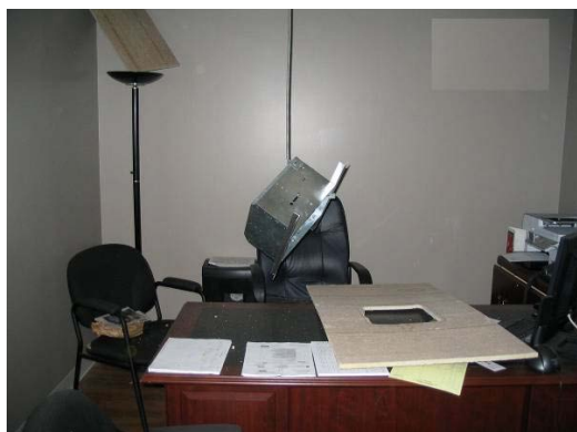
Figure 6. Neighboring business office damage
