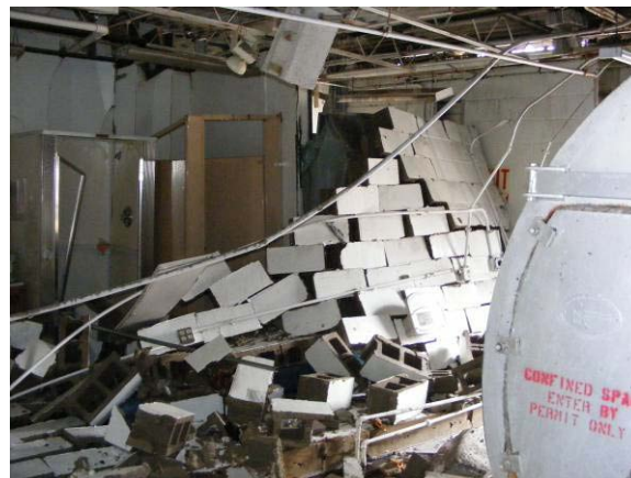
Figure 4. Boiler and locker room damage
