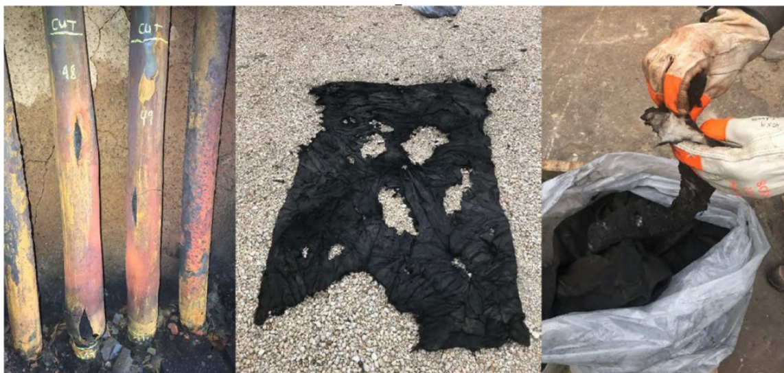
Figure 2. Failed fired heater tubes (left) and debris removed post-incident (center and right). (Credit: ExxonMobil)
