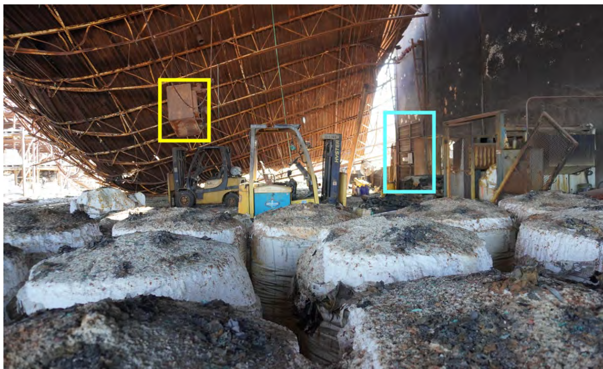
Figure 33. Super sacks located adjacent to the dock door (indicated by aqua box) and heater (indicated by yellow box) with the leaking vent penetration post-incident on October 14, 2024. (Credit: CSB)
