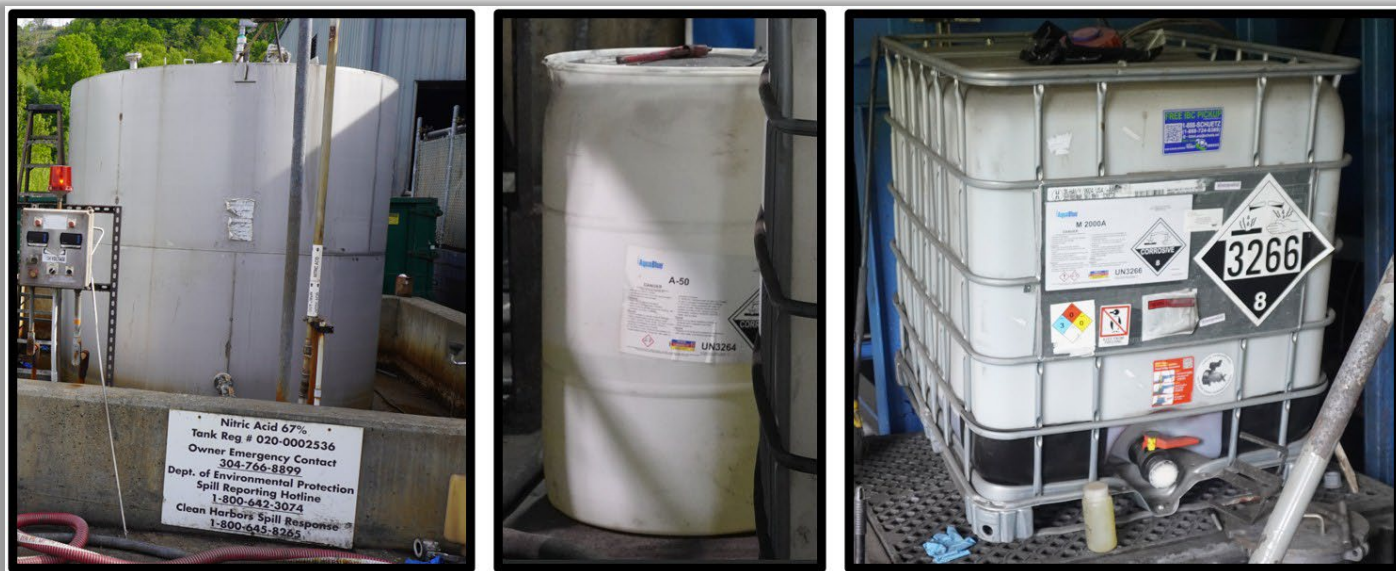
Figure 3. Nitric acid storage tank (left), A-50 drum (middle), and M-2000A tote (right). (Credit: CSB)
