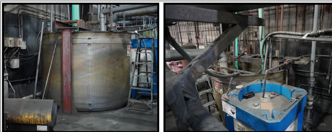
Figure 2. Incident tank, side view (left) and elevated view (right). (Credit: CSB)
