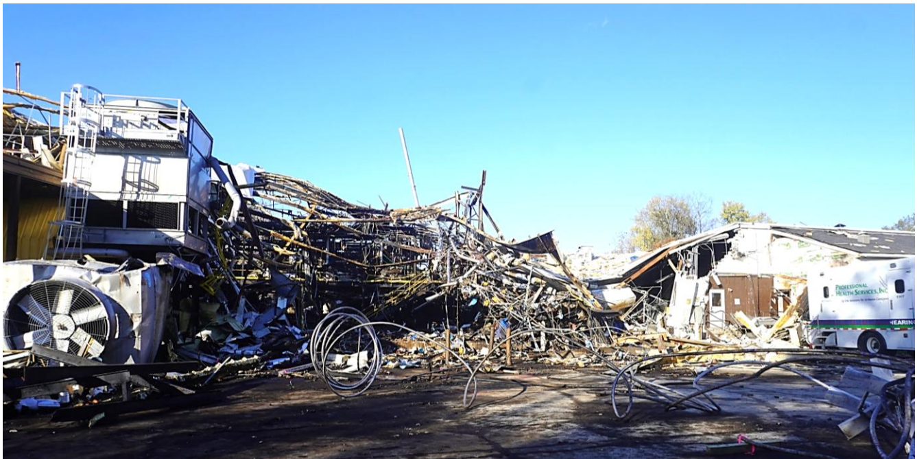
Figure 15. The Reactor 6 explosion destroyed the Louisville facility. (Credit: CSB)
