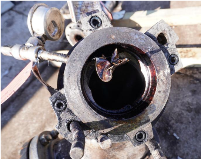
Figure 30. Reactor 6 rupture disc as found post-incident, fully open. (Credit: CSB)
