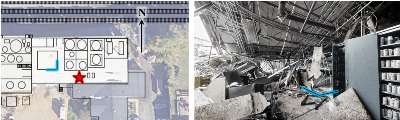
Figure 37. The collapsed control room at the Louisville facility after the incident. The red star in the left photo is approximately the camera perspective for the right photo, with the southeast corner of the control room indicated by blue highlighted lines. (Credit: Givaudan and Google Earth, annotated by CSB)
