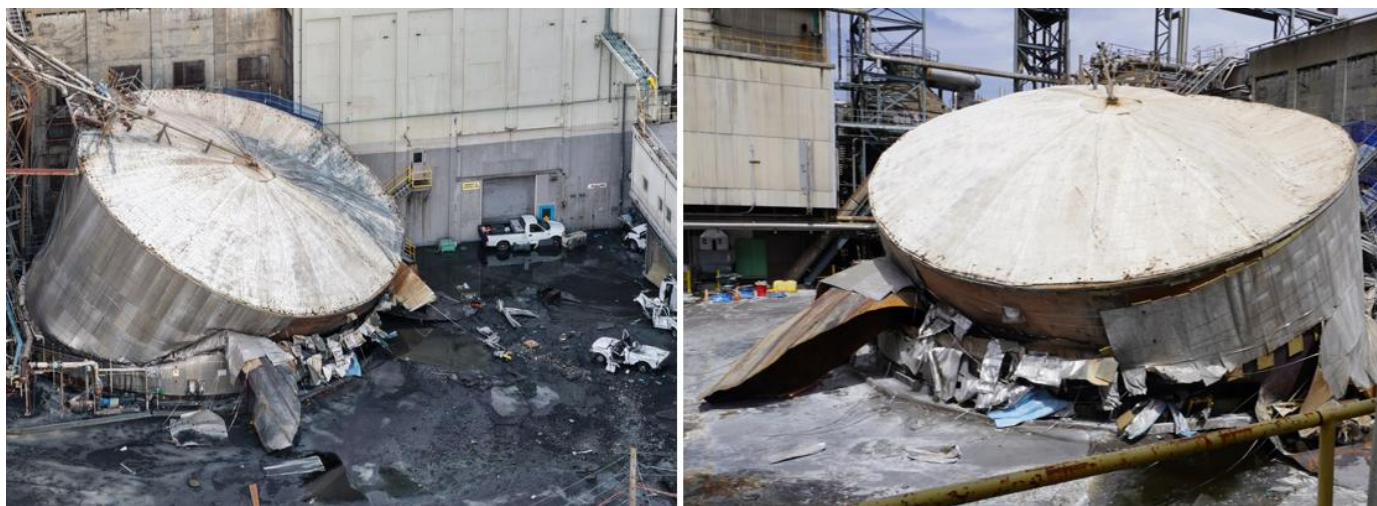
Figure 6. Post-incident photos of the failed G Tank at NDP in Longview, WA. (Credit Left: Seattle Times; Credit Right: CSB)
