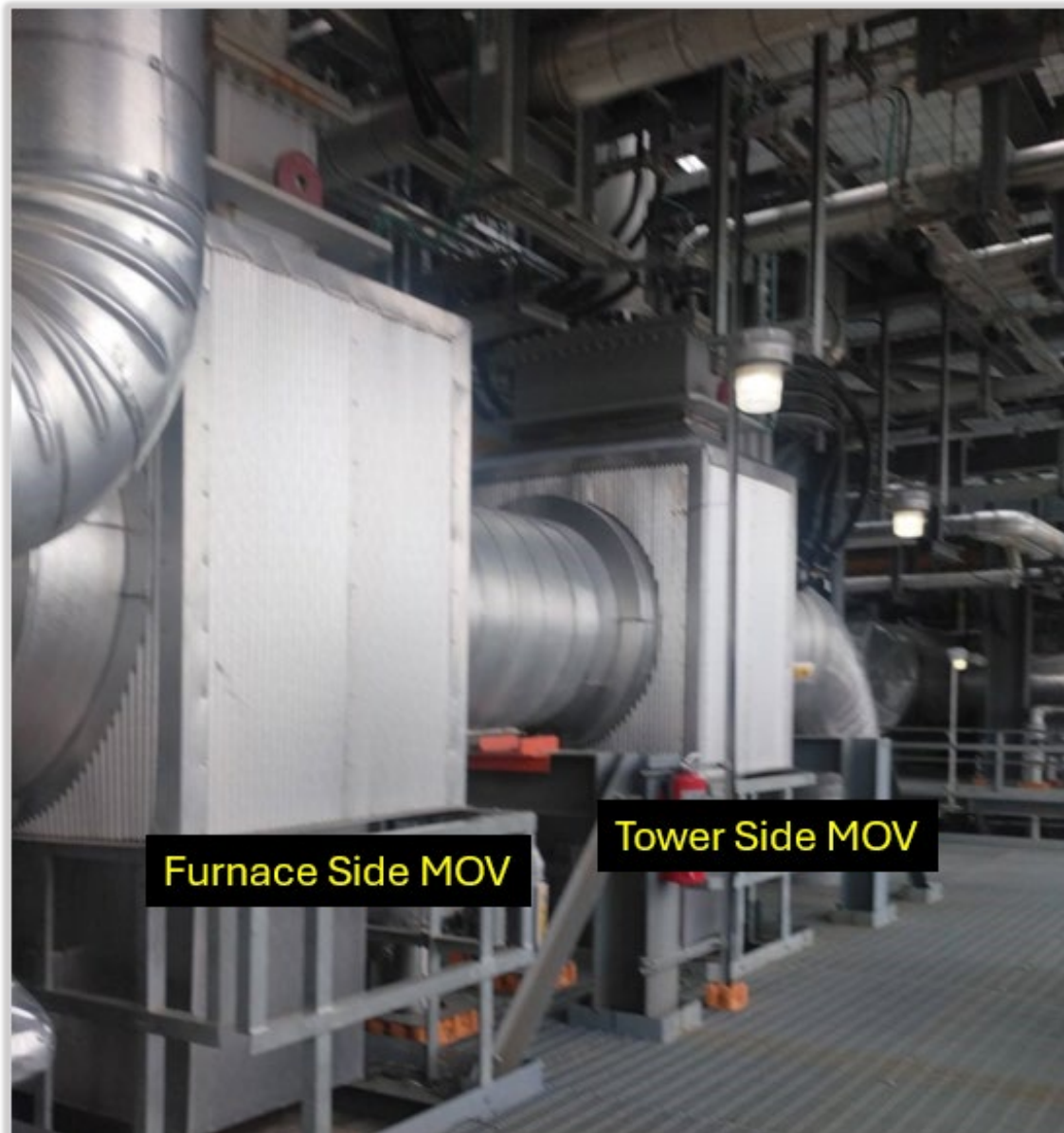
Figure 7. Furnace-side and tower-side 36-inch motor-operated valves after an ethane cracking furnace. (Credit: Shell, annotated by CSB)
