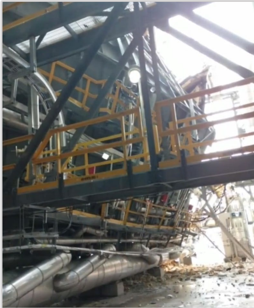
Figure 17. Furnace 5 after the explosion. (Credit: KDKA-TV)
