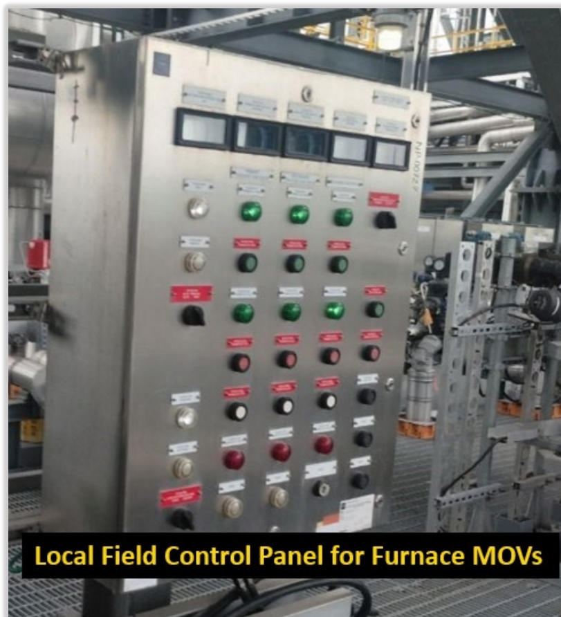
Figure 9. Local field control panel for furnace motor operator valves. (Credit: Shell, annotated by CSB).
