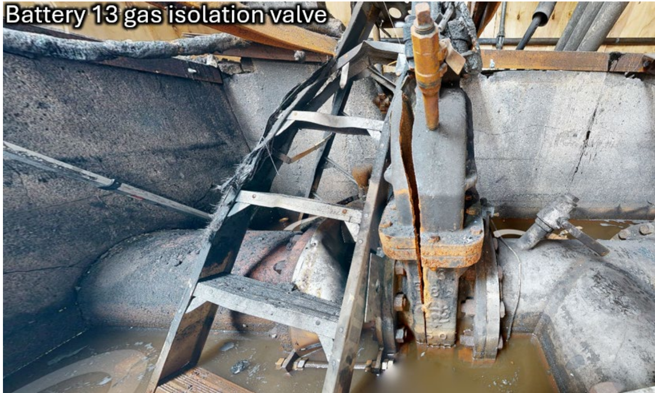
Figure 14. Photo of the Battery 13 gas isolation valve, as found after the incident. (Credit: Allegheny County Fire Marshal, annotated by CSB)
