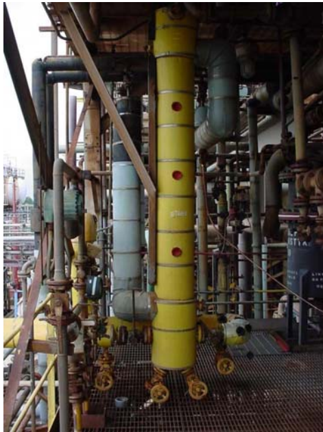
Figure 3. Vertical chlorine cooler in G-143a process.
