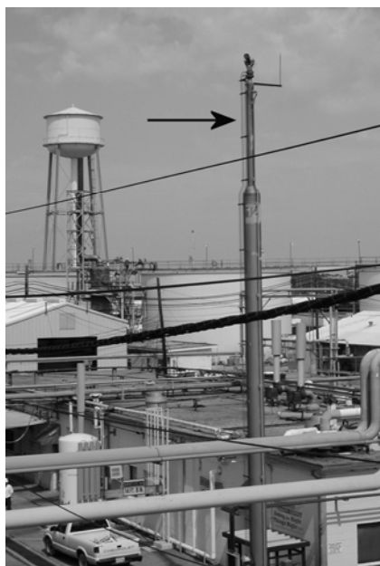
Figure 4. Typical water deluge tower.
