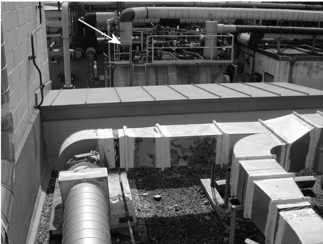
Figure 11. HVAC intake system on control roof (foreground).
