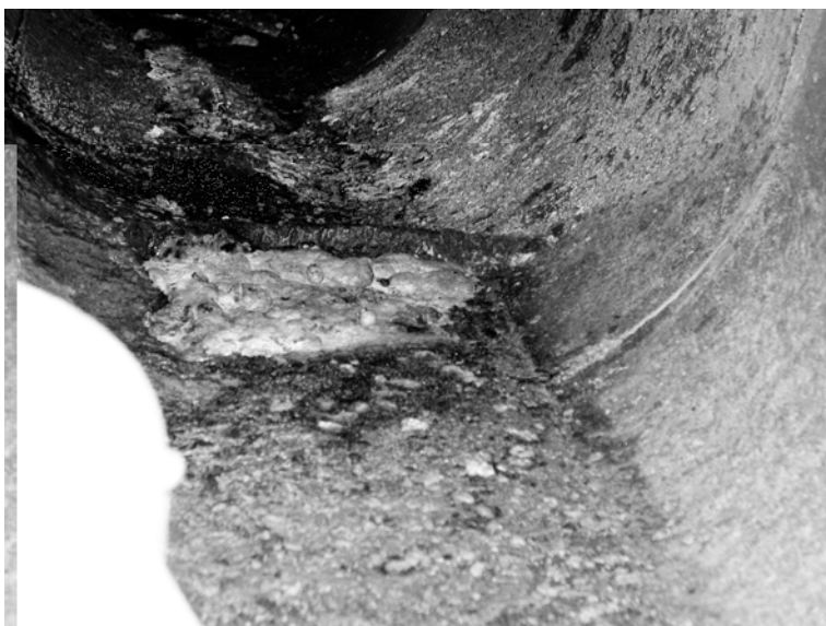
Figure 10. Solid deposits in main header duct.
