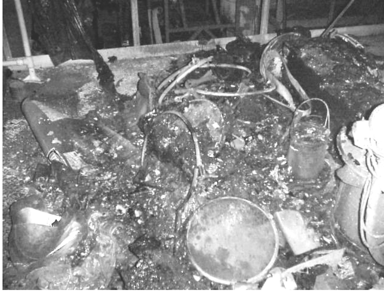
Figure 7. Remains of acid hood on mezzanine 1.
