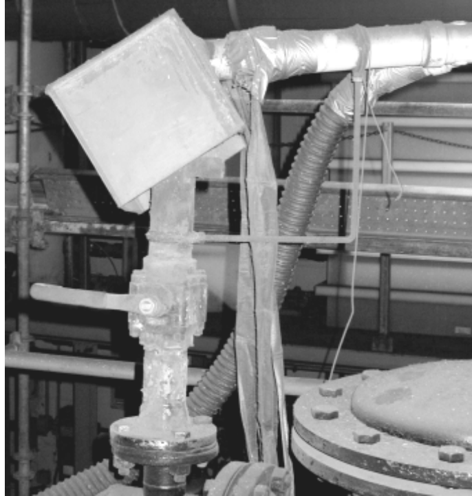
Figure A-1. Kestner unit exhaust ventilation.
