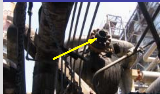
Figure 1. Carbon steel RHU heat exchanger outlet pipe (arrow) ruptured after operating only 3 months in high-temperature hydrogen service.
