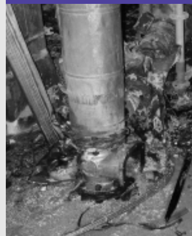
● Figure 1. Ruptured pipe/valve and fire damage.
