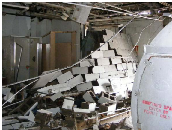
Figure 4. Boiler and locker room damage
