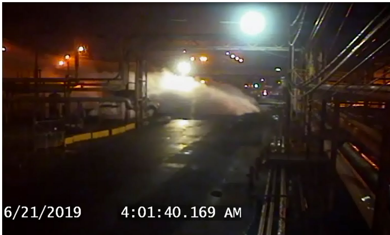
Figure 9. Security camera footage of leaking process fluid forming a large ground-hugging vapor cloud that surrounded some sections of the unit. (Credit: PES)
