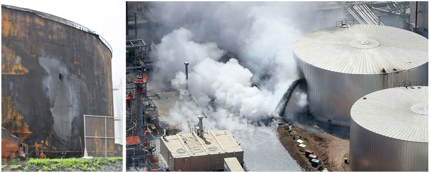
Figure 33. Post-incident photographs of the leaking asphalt storage tank at the Husky Superior Refinery. (Left photo credit: CSB. Right photo credit: Duluth News Tribune [50])
