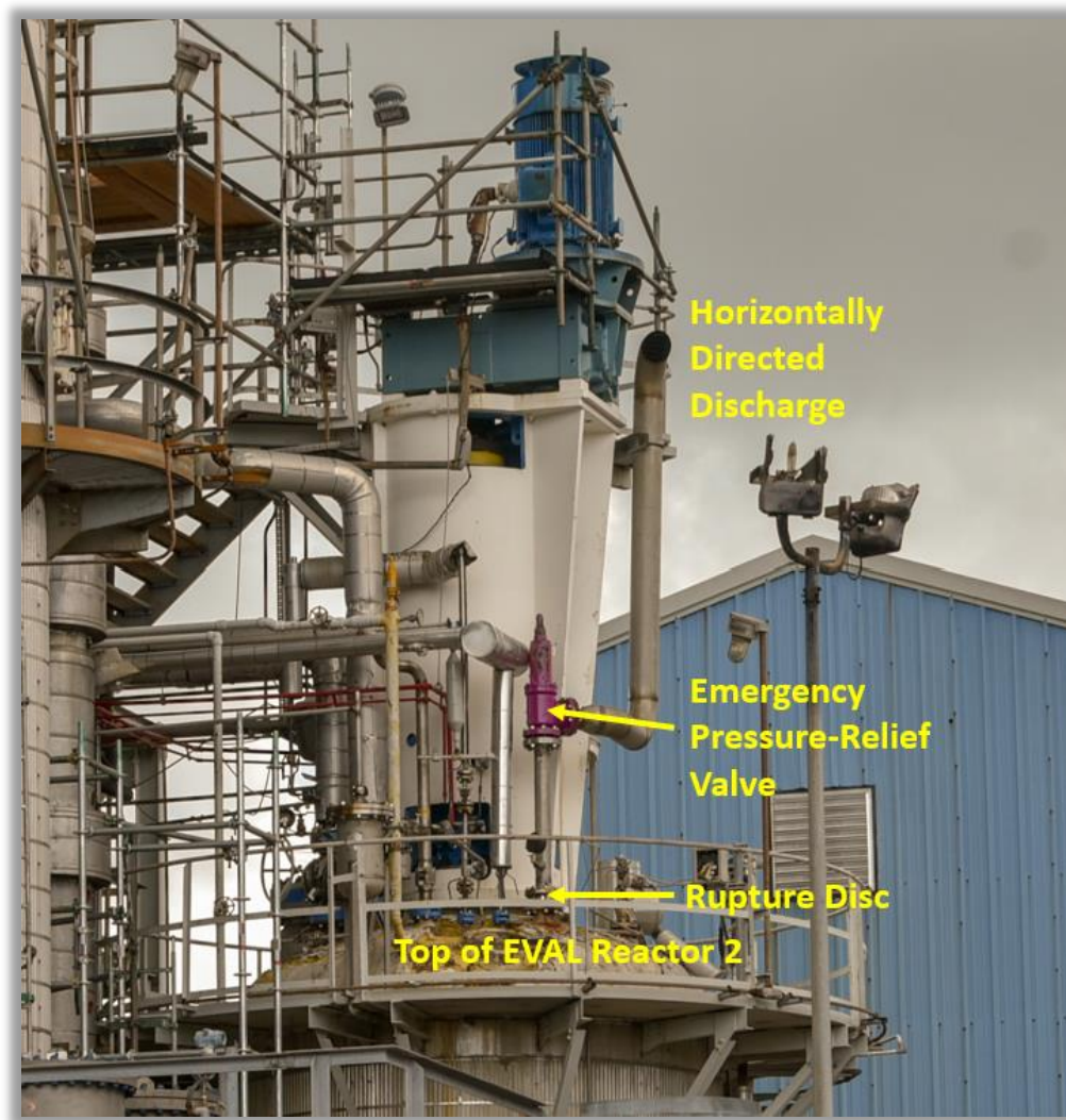
Figure 7. EVAL Reactor 2 Emergency Pressure-Relief System. (Credit: CSB)
