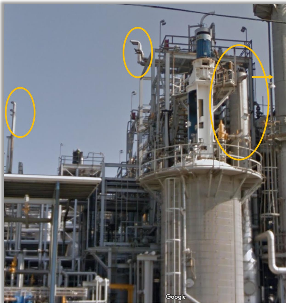
Figure 19. Horizontally Aimed Discharge Piping. (Credit: Google Maps annotated by CSB)
