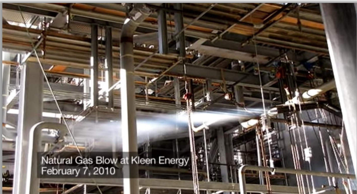
Figure 28. Horizontal Natural Gas Blow at Kleen Energy. (Credit: CSB [83])
