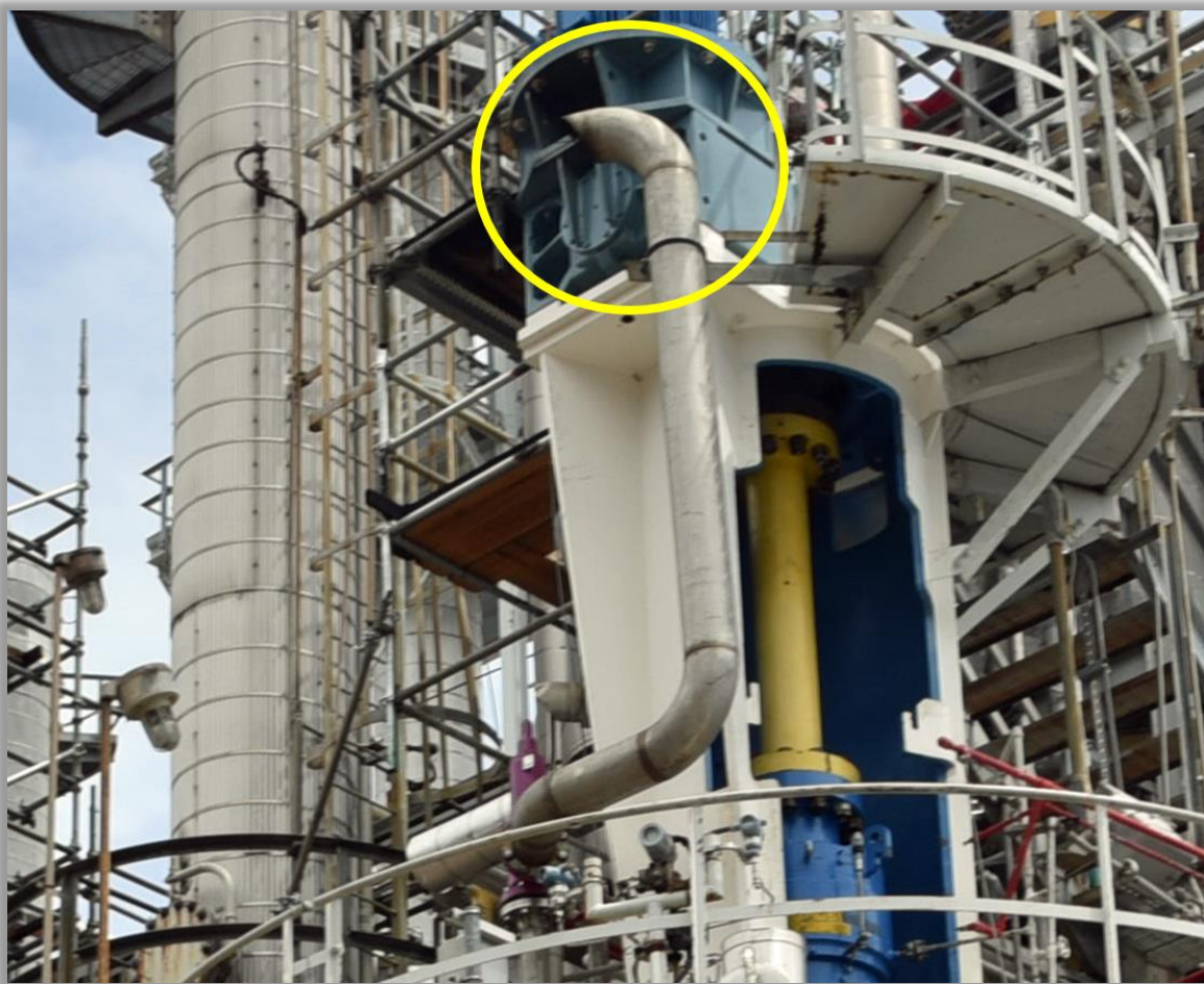
Figure 8. EVAL Reactor 2 Emergency Pressure-Relief System Outlet Piping. (Credit: CSB)
