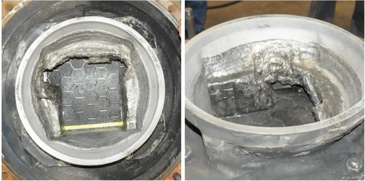
Figure 34. Spent catalyst slide valve view of the upstream side. (Credit: CSB)
