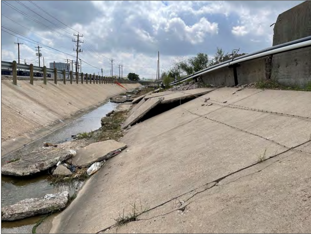
Photo 16: Damaged Section of Drainage Ditch, looking east
