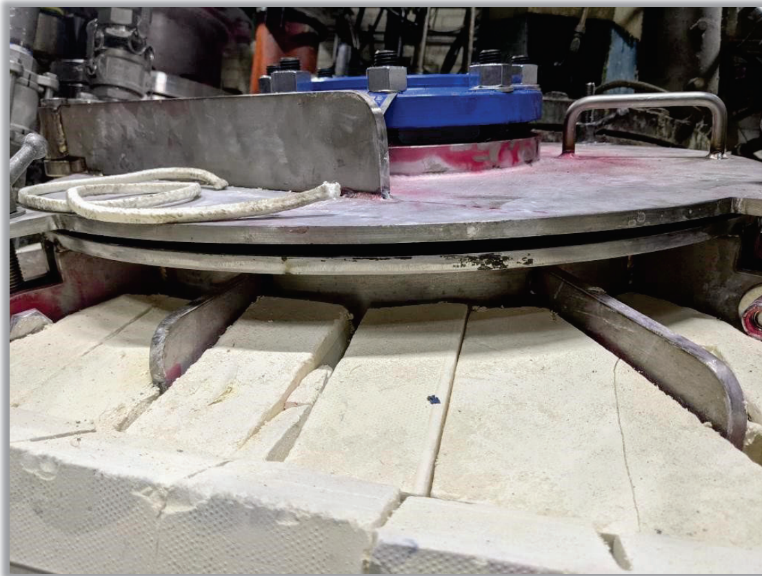
Figure 13. Bowing on the new manway lid in January 2021. (Credit: Yenkin-Majestic)
