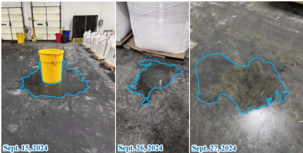
Figure 32. Roof leaks discovered in the Plant 12 Storage Warehouse on September 15, 26, and 27, 2024, with each puddle extent outlined in blue. (Credit: KIK, annotated by CSB)
